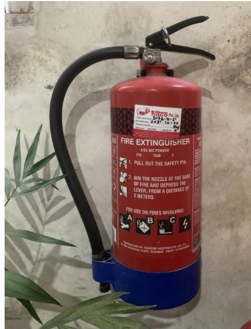
Figure 2: Fire Extinguisher inside office area
